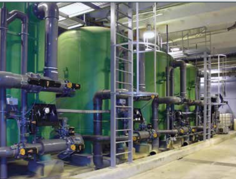
Continuous-flow adsorber in a water treatment plant
