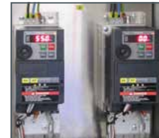
Frequency converters for controlling the pumps
