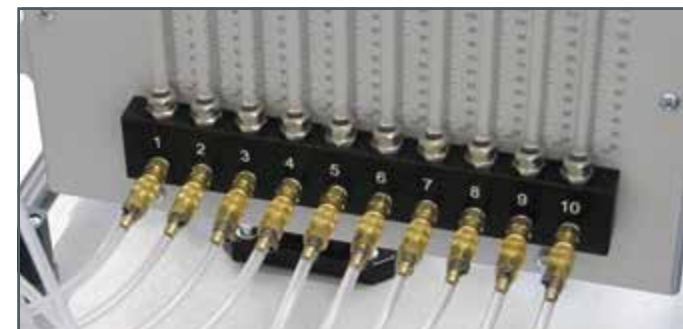
Connections on the manometer panel for measuring the pressure in the filter bed
