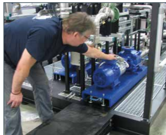
Pumps can be removed and tested
