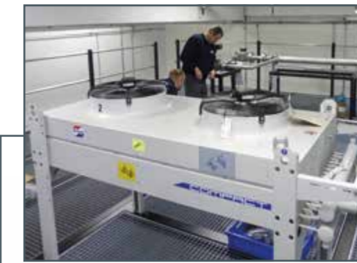
Dry cooling tower
