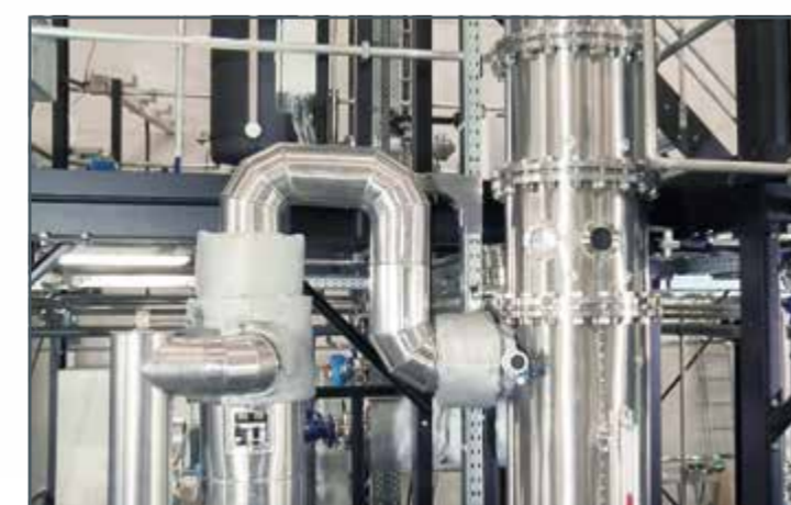
Steam supply for distillation process
