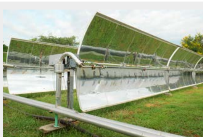
For a power plant, individual parabolic trough collectors can be connected in a collector field.
