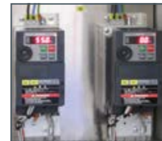
Frequency converters for controlling the pumps
