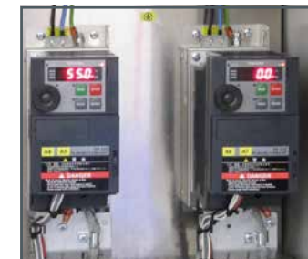
Frequency converters for controlling the pumps
