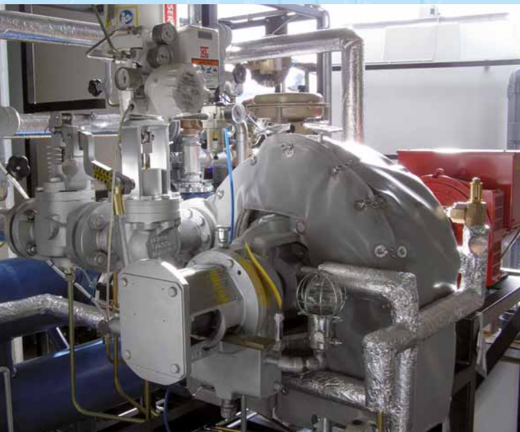
Steam turbine with throttle valve and generator (background)
