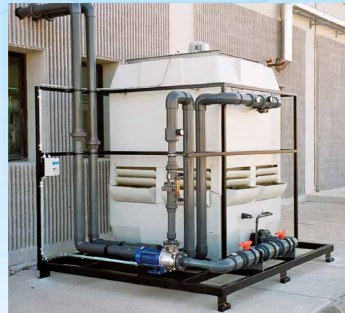
Wet cooling tower with cooling water pump
