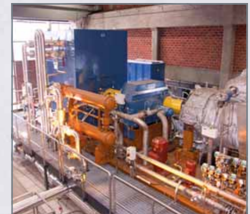
Steam turbine system for a paper mill
