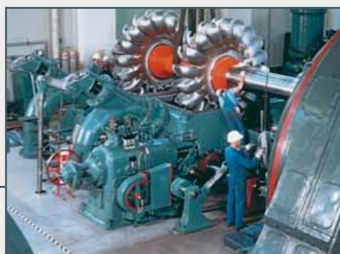
Assembly of a Pelton turbine at the Walchensee power plant in Germany (Voith Siemens Hydro Power)
