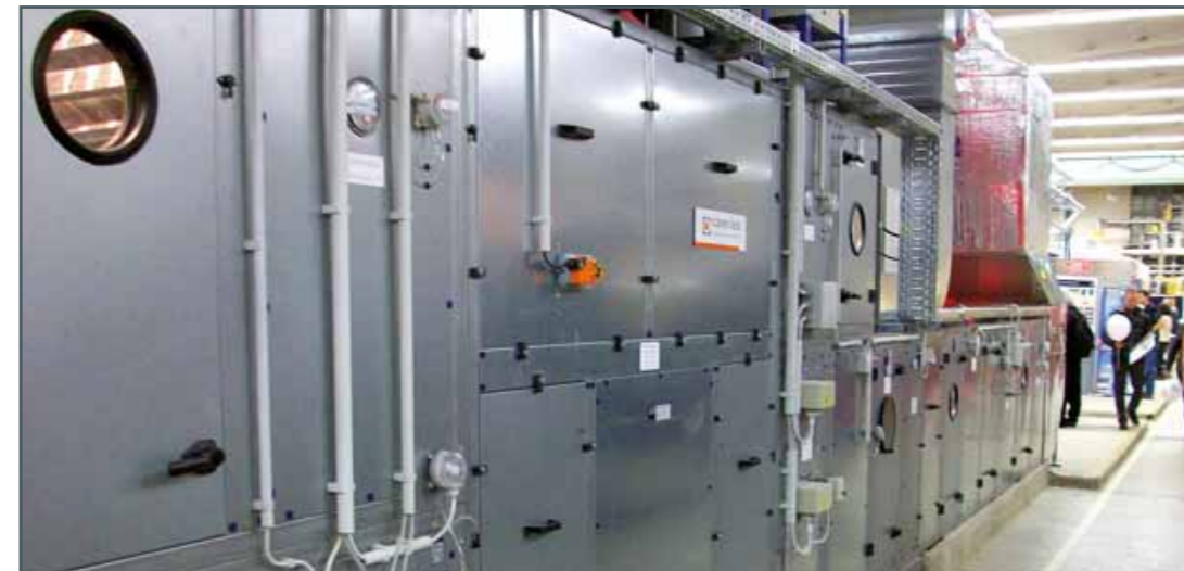
An example from practice: industrial air conditioning system with comprehensive filters for clean room production
